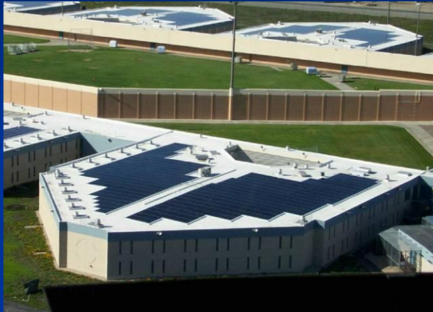
1.2 MW Solar PV (Existing)
