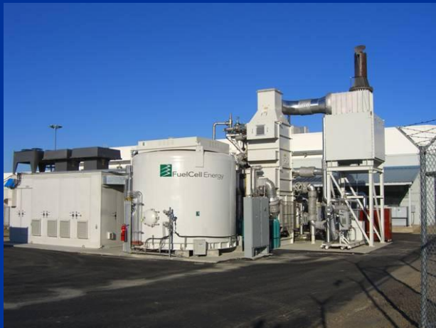
1.0 MW Fuel Cell (Existing)
