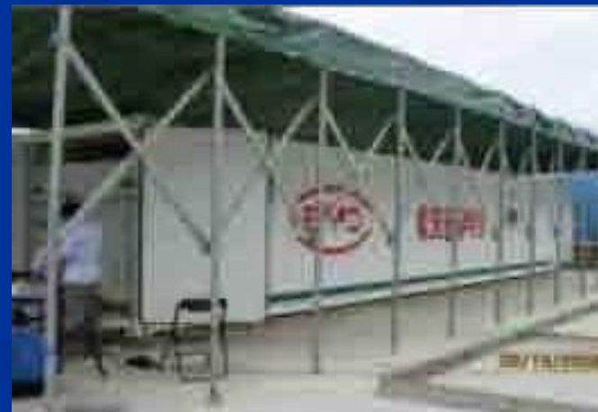
2.0 MW Advanced Energy Storage (New)
